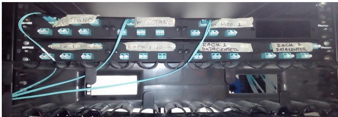
Figura 6. Cassette de fibra rack data center
